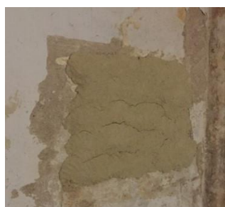
Figure 2: Compress material on salt contaminated masonry.
